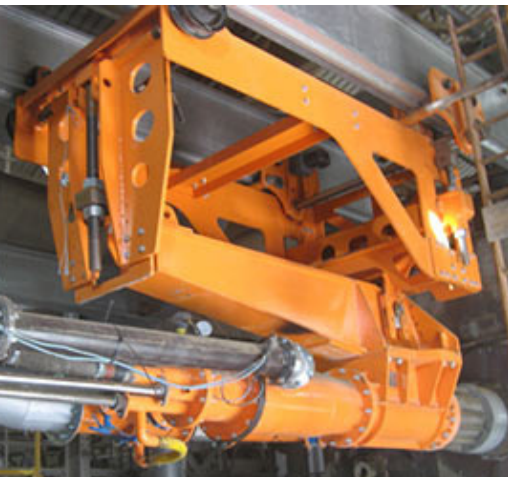
Burner with mounting arm supported from motorised overhead trolley
