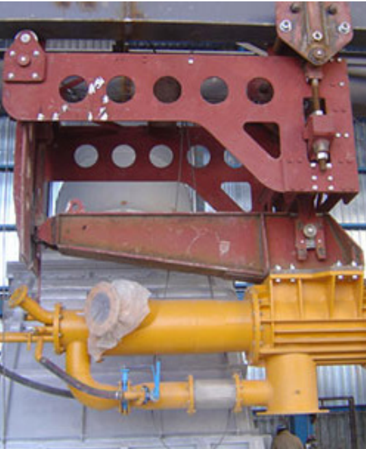
Large rotary kiln burner supported by overhead trolley
